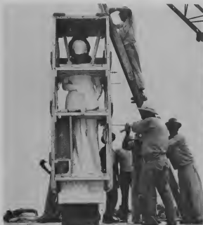
Set in its permanent position, workmen remove the many nuts, bolts and bars that held the statue rigid. It arrived without a single mark. Poni na su posicion permanente, trahedornan ta kitando e hopi nutnan, boltman y baranan cual a tene e estatua pa no mové.
